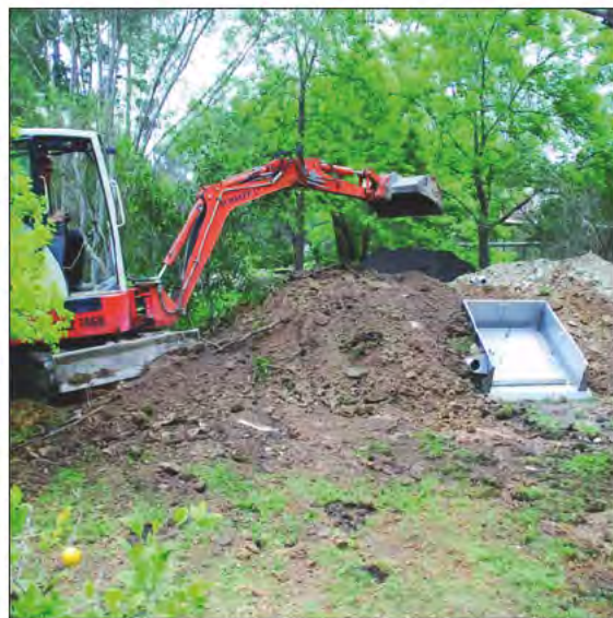
Avoid heavy machinery close to the edges of the bunker.
